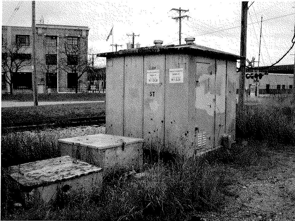
PC030021 Looking north from park property toward Baldwin Street and and closeup of Wisconsin and Southern railroad facilities adjacent to park property.
